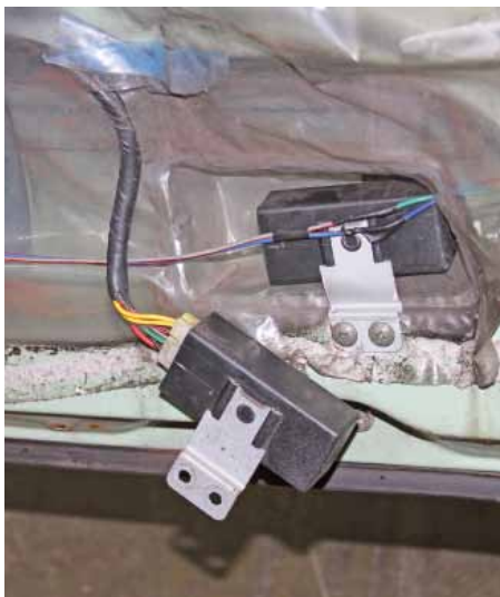
6 The contacts on this can corrode, but it is very hard to open and close the unit to access them for cleaning. So we tested it by substituting another relay. That did the trick, and that was duly fitted.
